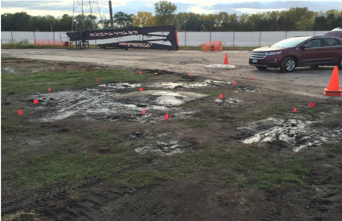
Photo 4: Area 2 Injection Array and Monitoring Wells
