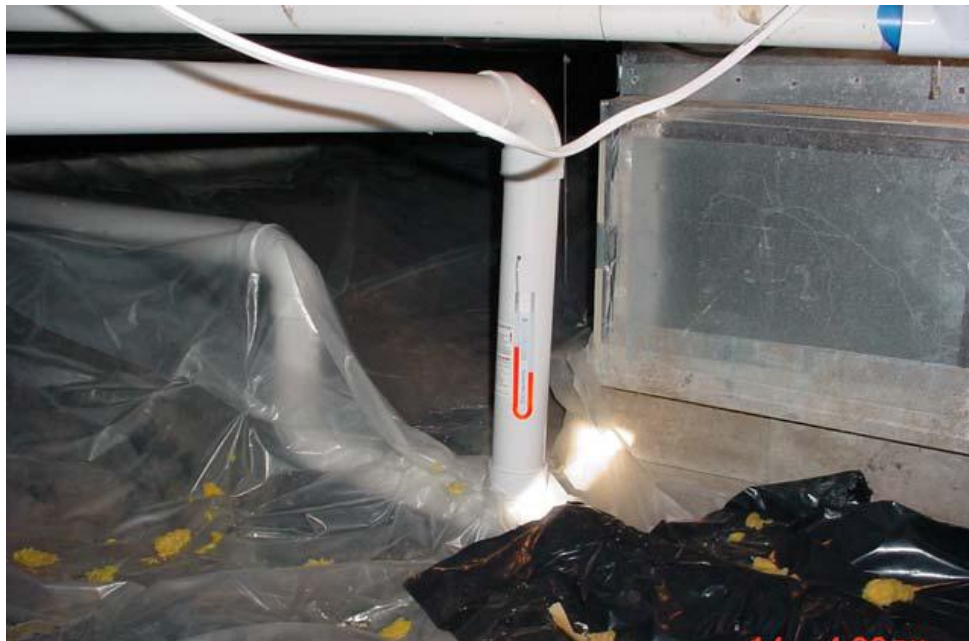
Figure 14-3. Crawl Space Mitigation Using SMD (Source: ITRC, 2007; Courtesy of Kansas Department of Health and Environment)
