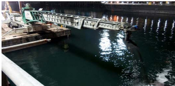
Conveyor system distributing in berthing area
