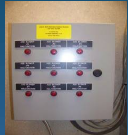
Low Pressure Monitoring Panel Courtesy Tom Hatton, Clean Vapor, Inc.
