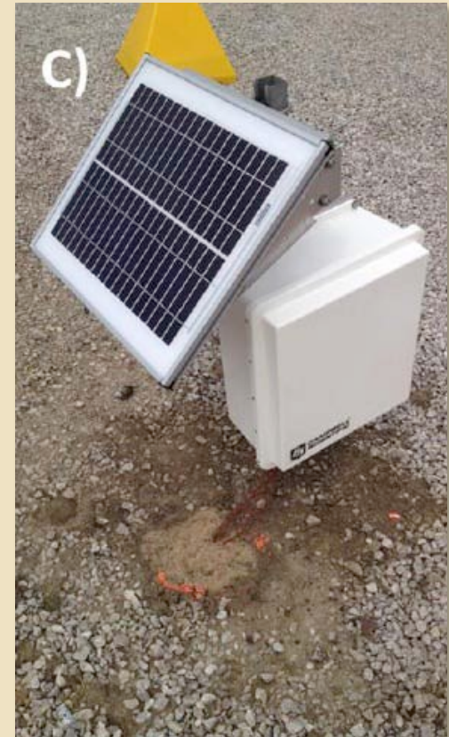
Solar power supply and weatherproof box with data logger and wireless communications system.
