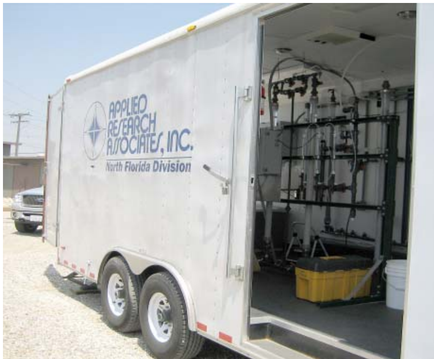
ARA Demonstration Trailer Containing Ion Exchange Equipment at Well-Site F-17 in Fontana, California.
