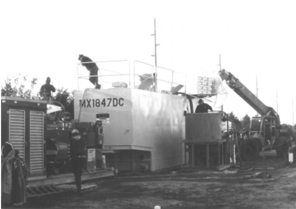
Figure 4. Bulk materials handling, slurry mixing, and high pressure pumping systems.
