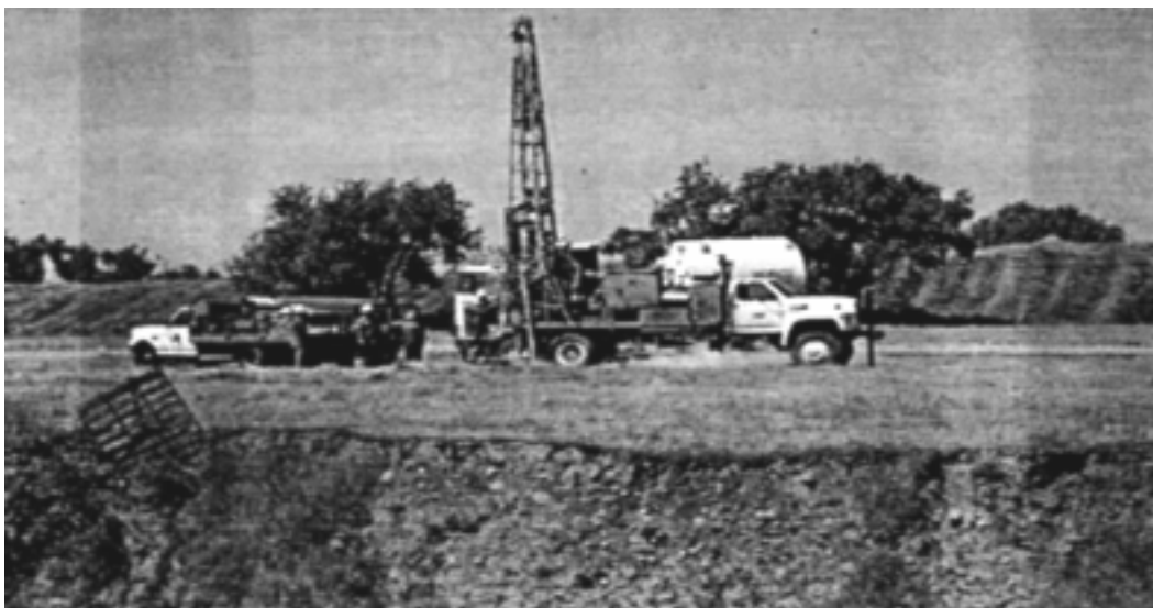
Figure 6. A cryogenic drilling site. Large boulders in the subsurface, visibly exposed in the trench in the foreground, do not present a drilling challenge using this technique.
