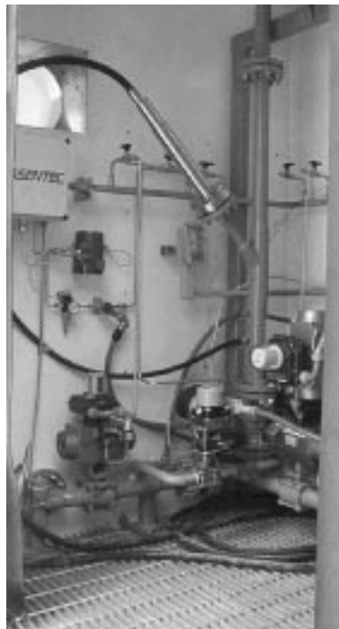
Figure 2. Lasentec M600P analyzer installed in GAAT Slurry Monitoring Test Loop.
