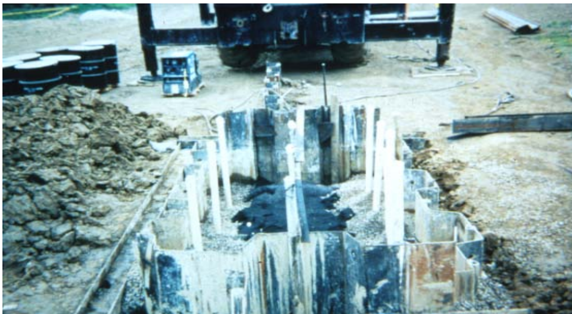
Figure 7-2. Photo of a pilot-scale monitoring system, New York (prior to sheet pile removal to create a flow-through gate section).
