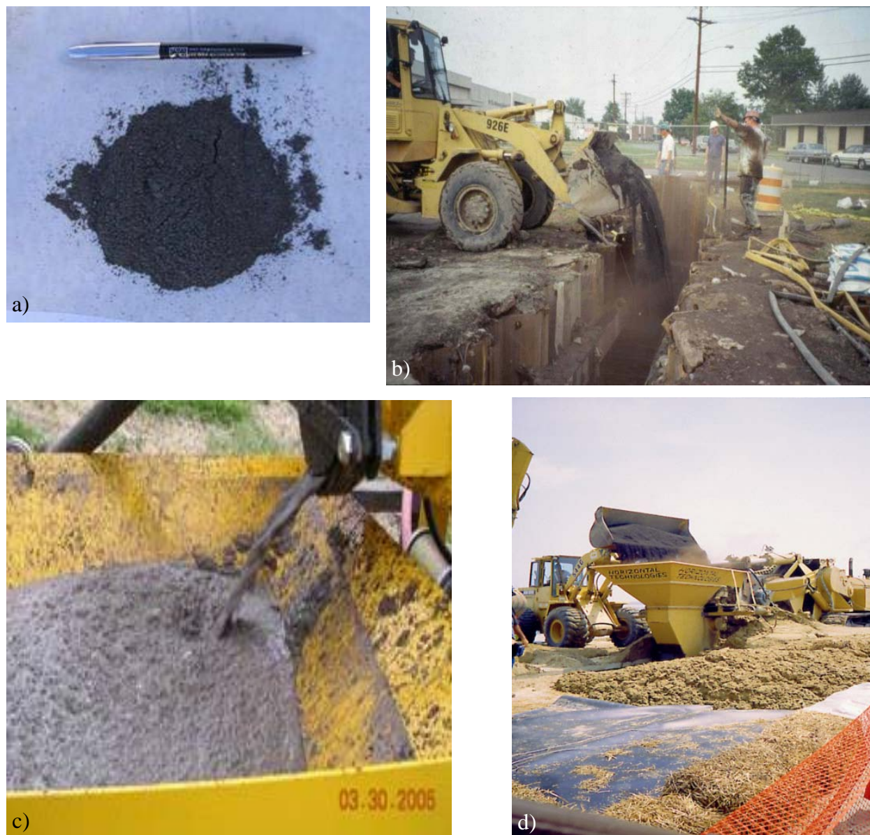
Figure 4-1. Examples of ZVI and ZVI emplacement: (a) fine-grained ZVI, (b) coarse-grained ZVI being placed in a trenched PRB, (c) microscale ZVI in an injectable EHC ® slurry, and (d) installation of ZVI PRB at a U.S. Coast Guard facility using a one-pass trencher.
