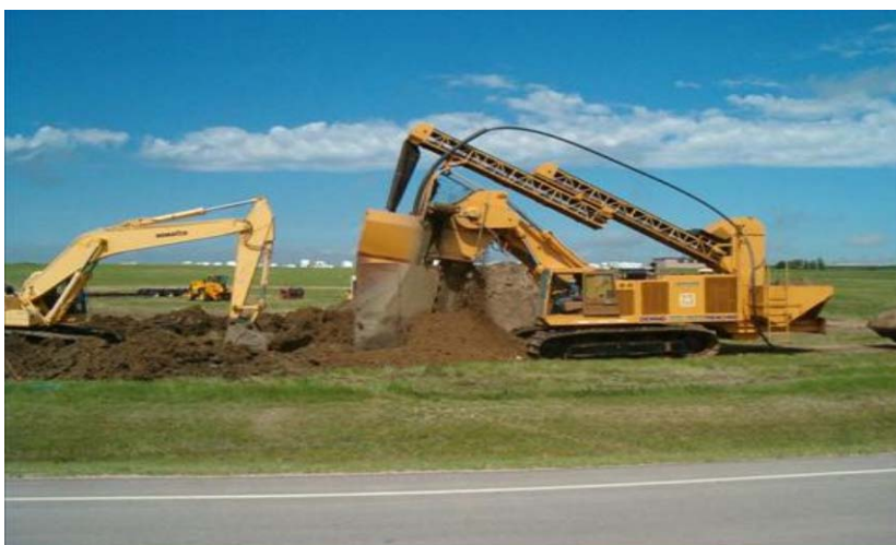
Figure 6-3. Continuous chain trencher at Ellsworth AFB, South Dakota. (Courtesy of the U.S. Air Force)
