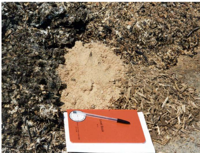
Figure 4-6. Materials used in construction of the OU-1 biowall, Altus Air Force Base, Oklahoma.
