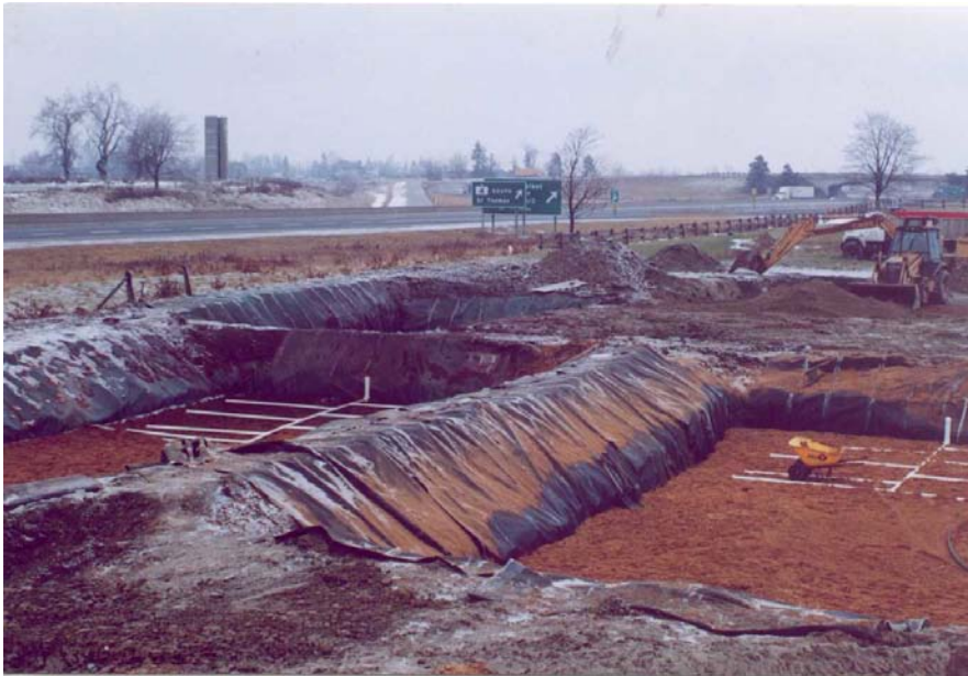
Figure 6-1. Horizontal PRB for treatment of septic system nitrate. (Courtesy of Septech, Inc., 2003)
