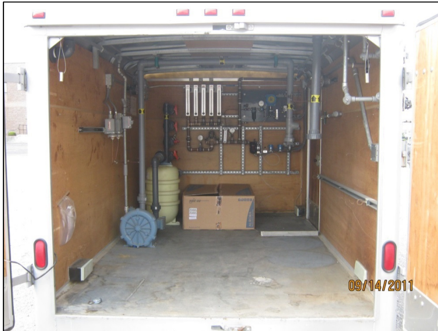
Figure 5-20. Inside of Trailer # 2, which houses the propane feed and distribution as well as SVE equipment.
