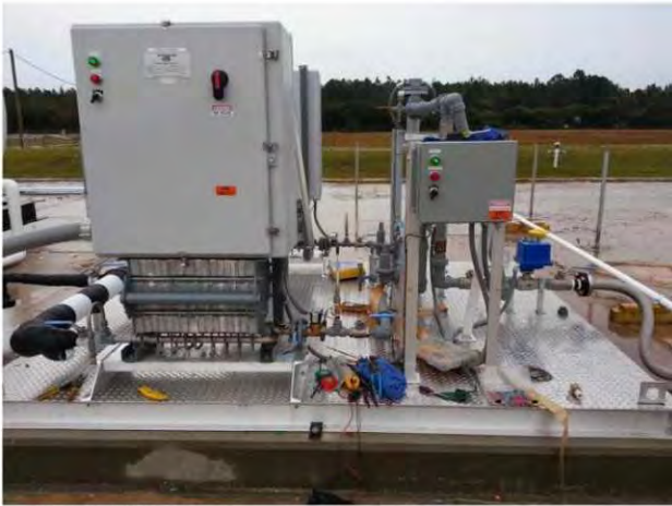
Left: 105-kW process vaporizers.
