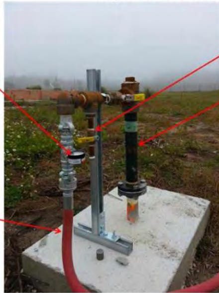
Above: Typical distribution panel. Below: Typical sparge wellhead installation
