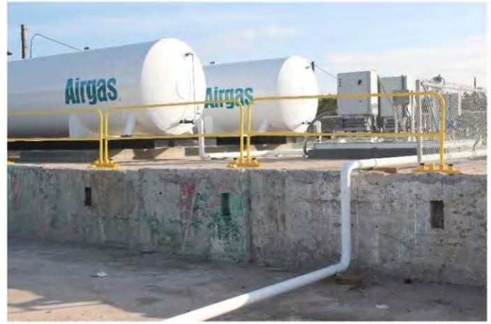
Right: 50-ton CO 2 storage tanks
