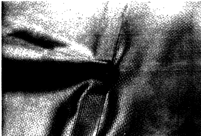
Figure 10.2(a). Formation of "fishmouth" resulting from excessive slack in upper geomembrane versus lower geomembrane
