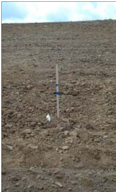
Figure 5-5. Intermediate cover layer at Denver Arapahoe Disposal Site, grade stake marked for placement of other layers.
