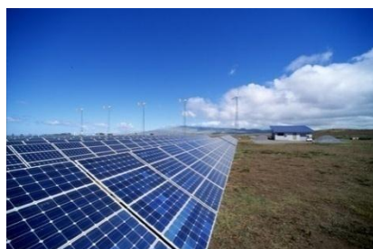
Source: NREL PIX 13823
