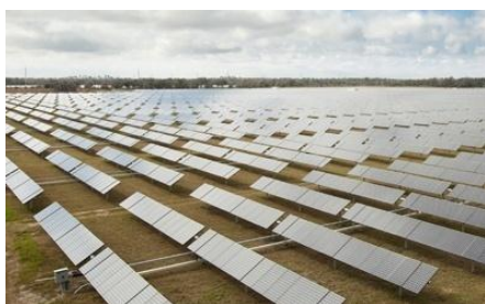
Source: SunPower Corporation
