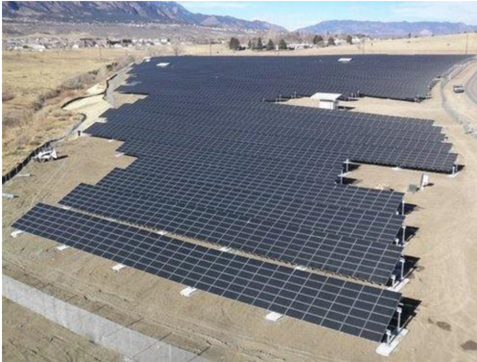
Source: NREL PIX 17394
