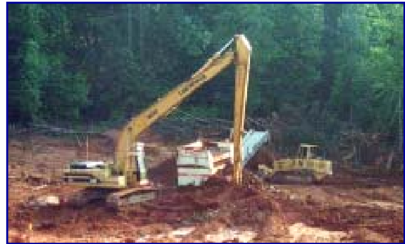
Tele-operated Caterpillar 325L Excavator and Caterpillar D8 Bulldozer Photo courtesy of the U.S. Air Force Research Laboratory
