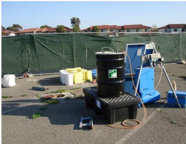
Figure A-1. Solar Powered Skimming System for LNAPL Recovery (see blue equipment)
