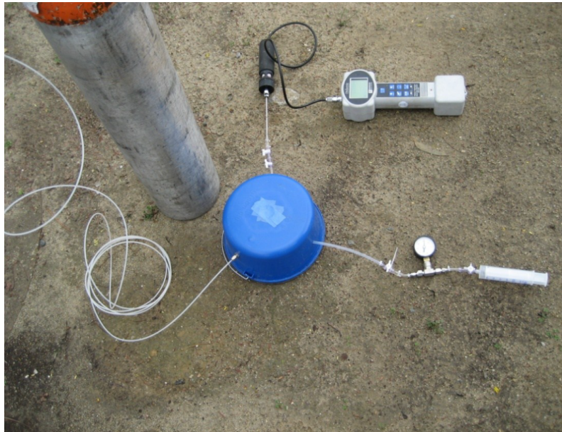
Figure G-13. Gas shroud over Vapor Probe Surface Completion. System consists of shroud (blue bucket), helium cylinder, field helium detector and syringe with vacuum gauge for purging.
