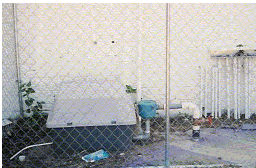
Figure 6-1. Small-scale SVE system designed to address the source of vapors and protect the on-site building. The housing contains a small SVE blower that services SVE wells and was not designed to address the entire source of vapors.
