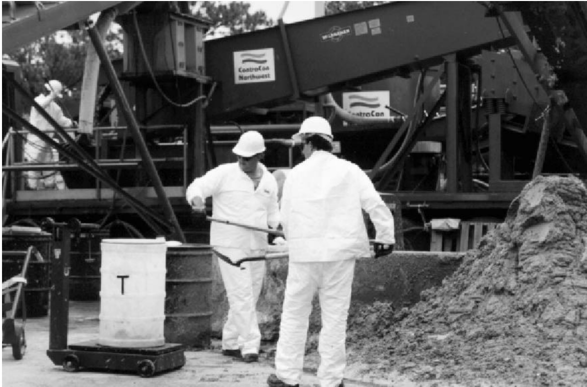
Figure 17. Collecting a 150- to 300-lb sample of processed soil (T) for verifying process efficiency.
