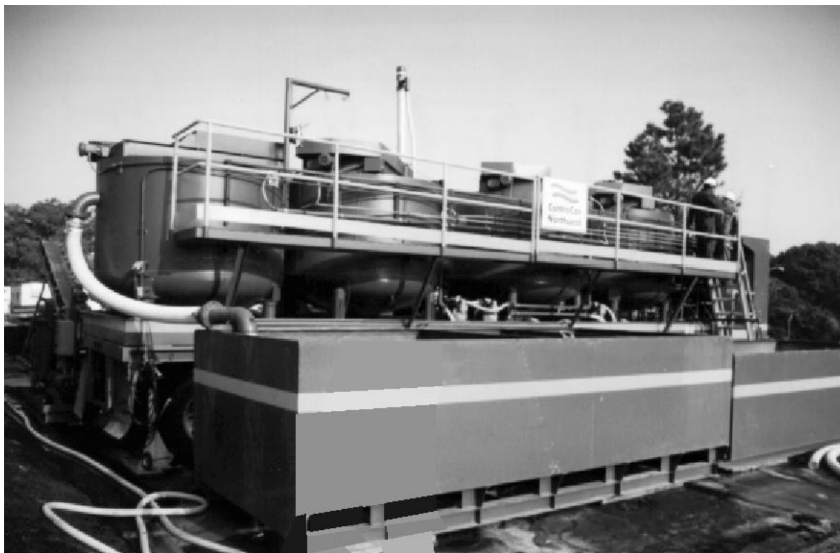
Figure 10. Leaching and precipitation tanks and clarifiers that were part of Vendor 1's plant.
