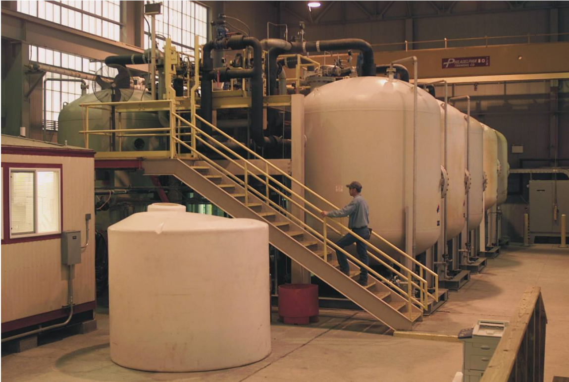
Fig. 5. Photo of the Fernald Site Treatment Plant, Showing Resin Vessels
