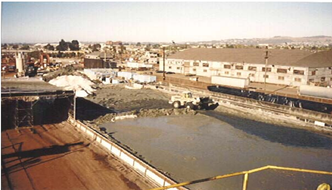
Figure 4-5. Dewatering and Pretreatment Facility for Dredged Sediment
